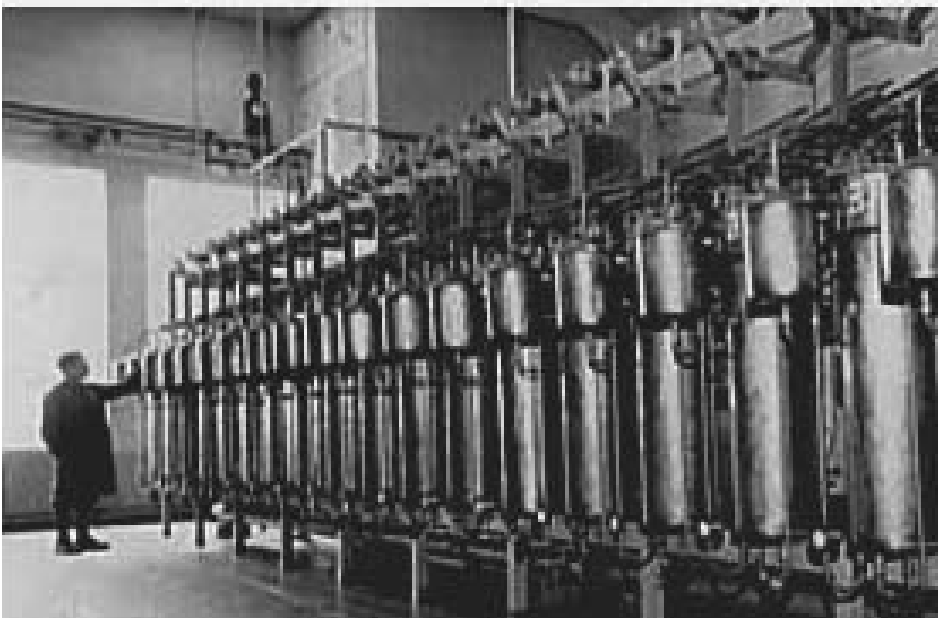
The heavy water collectors at Vemork
